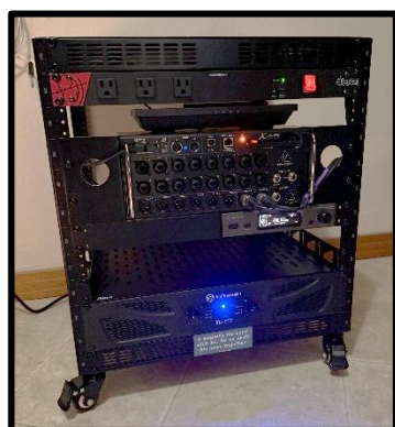
Network rack with new mixer
